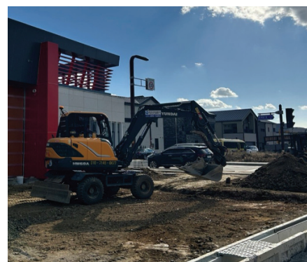
Fig. 6. Absence of danger sign
