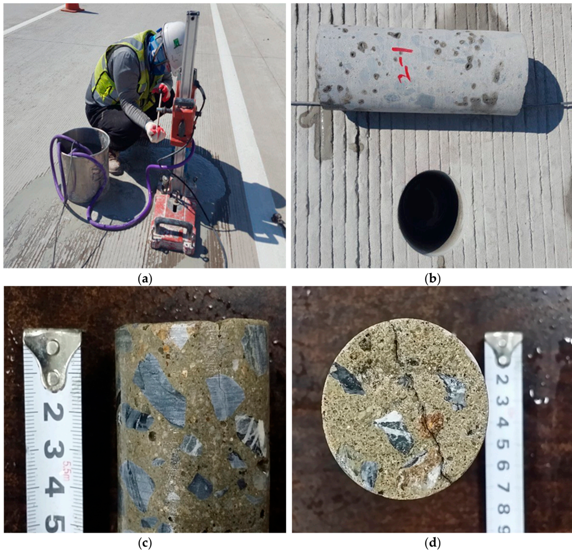
Figure 4. Preliminary field study (2017) on the Gwangju–Daegu expressway, Republic of Korea. (a) Coring operation at the site, (b) core sample, (c) crack depth, and (d) surface crack of the core sample.
